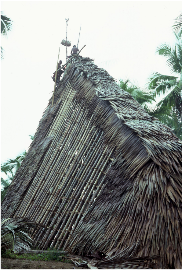
69. The thatching of the roof of a ceremonial house. Kumunware hamlet, Wainakim.
