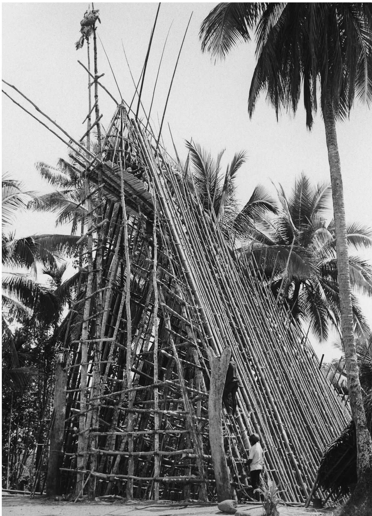
28. The construction of a ceremonial house in Waignakim. The crucks and rafters are leaning against the scaffold inside and the ridge beam above.
